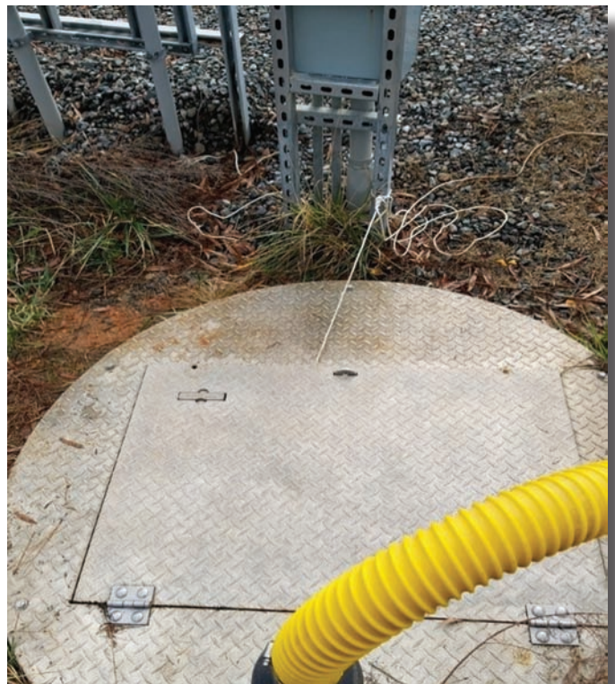
OdaLog® Sulfide Monitor suspended into manhole to determine H 2 S levels.
